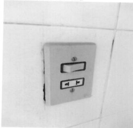
Interruptor e tomada
